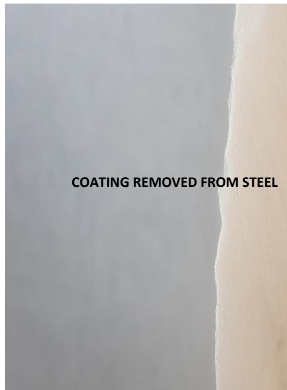
Figure 12: Coating removed from steel
