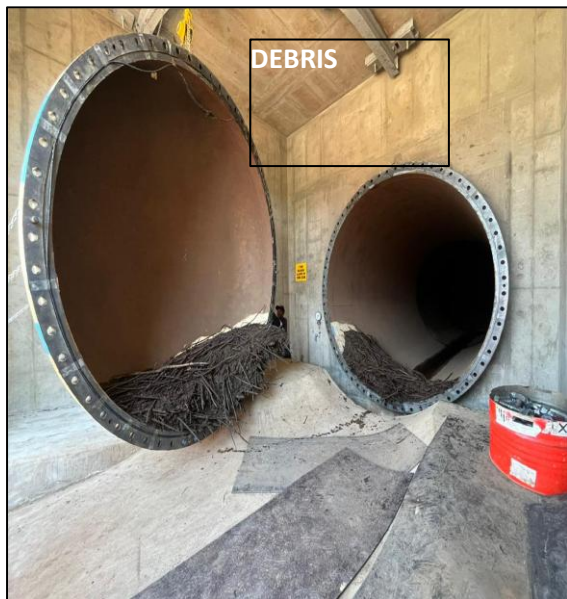
Figure 15: debris inside the tunnel
