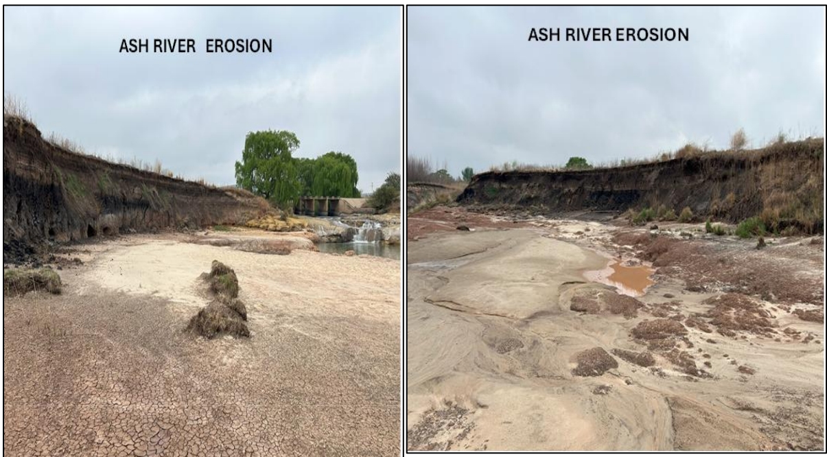
Figure 18: Ash River Erosion
